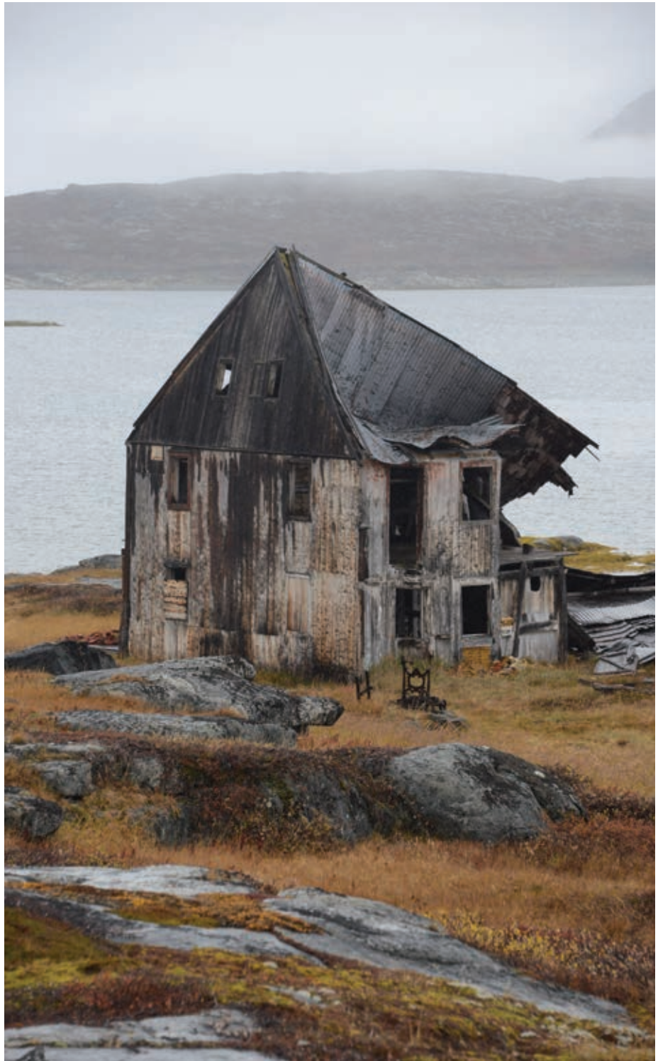
Derelict buildings collapsed from age at the Moravian Mission in Hebron Fjord, Labrador.
